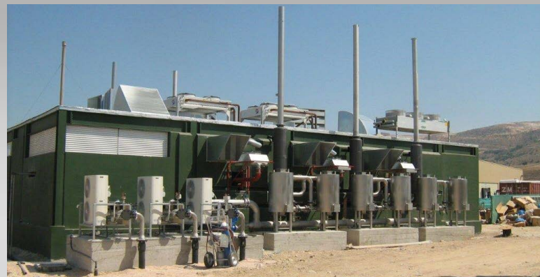
Seven CHP with an installed capacity of 1.8MW produce electricity and heat.
