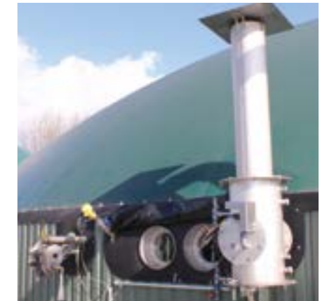
Gas storage & control unit
