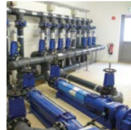
Central pump block
