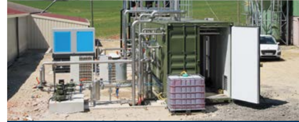
Top: In Jeppo (Finland), the biomethane gas station is open 24/7.
