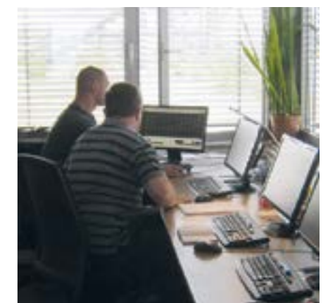
Process control system
