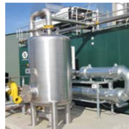
External gas desulphurisation
