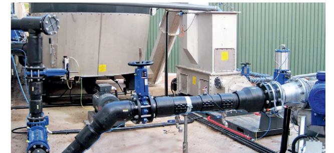
Positioning of MULTIMix between the solids input system and the fermenter.
